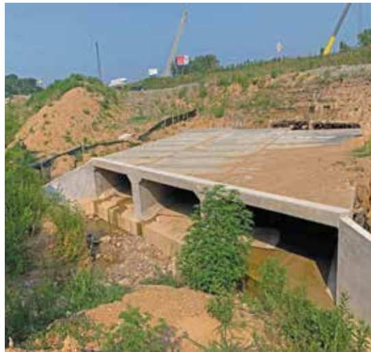
IMPROVED FLOW The new triple-barrel box culvert provides more flow for creek water. The crew also installed head and wing walls on both the north and south sides of the culvert.
